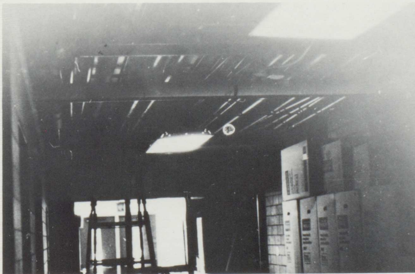
With the ceiling tiles out, it made walking through the halls seem like crawling through a cave.
